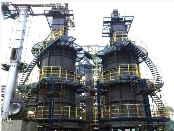
蒸汽过热炉 Steam superheater
