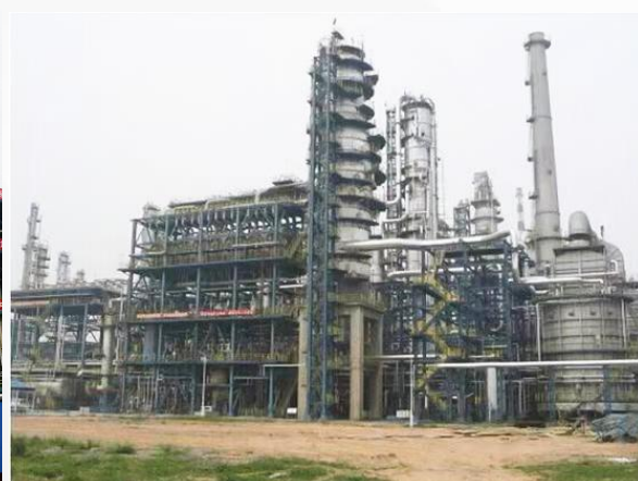
重整加热炉 Reforming furnace
