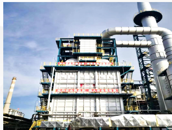
进料加热炉 Feed heating furnace
