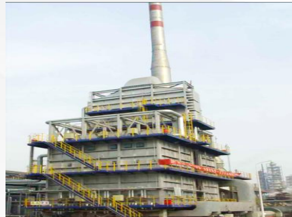
醋酸裂解炉 Acetic acid cracking furnace
