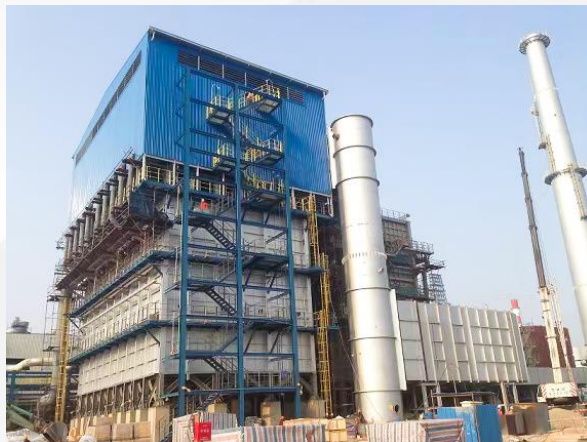
制氢转化炉 Hydrogen producing reformer
