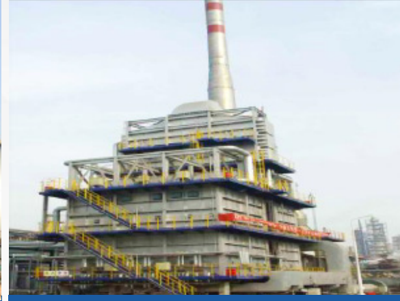
Acetic acid cracking furnace
