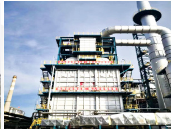
Feed heating furnace
