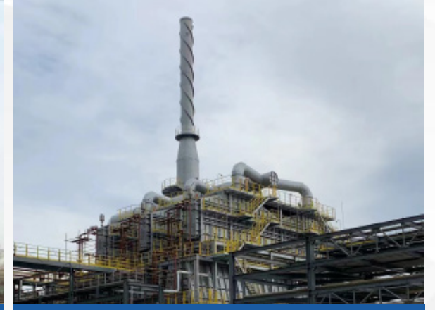
Needle coke heating furnace
